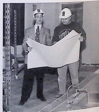
Looking over the SLC renovation plans are Robert Saffian, Wilkes staff architect, and Mike Hardik, job coordinator, Power Builders, Inc.
