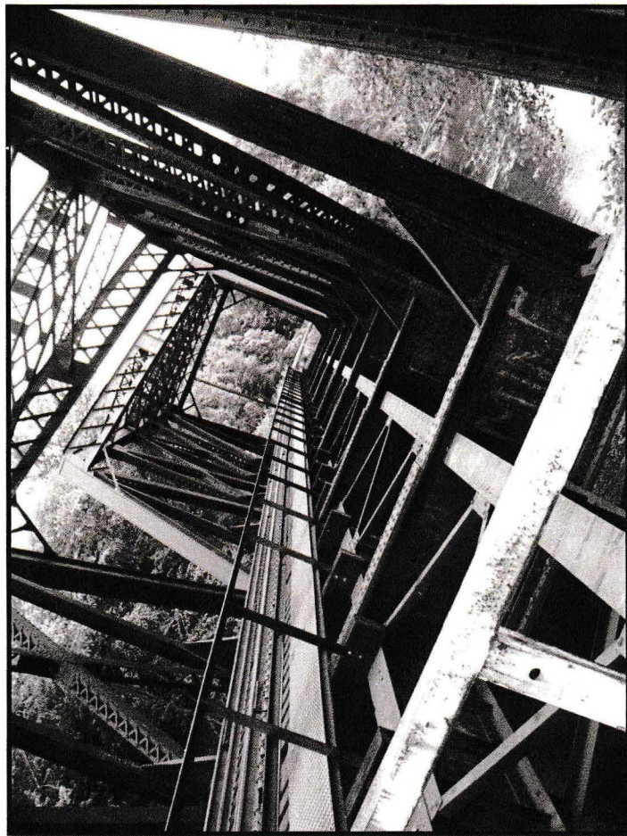
THE RUSTED RAIL
