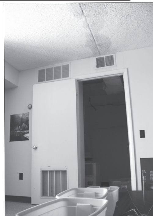
The Beacon/Jenna Stephens Buckets catch water leaking from the ceiling of apartment 670.
